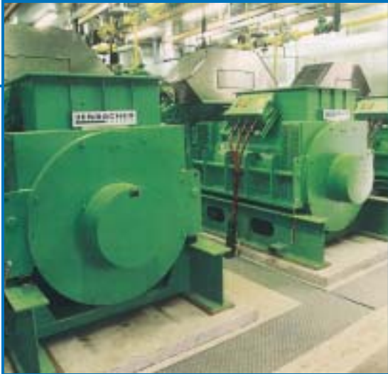
Natural gas cogeneration modules
