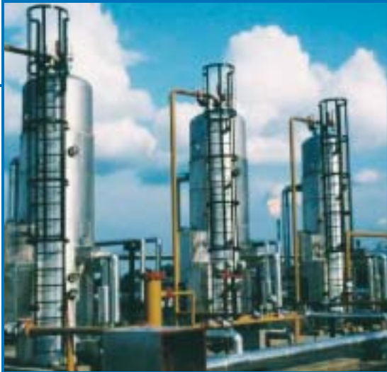
The NIS Refinery
