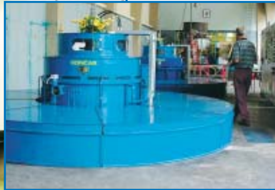
Generators in the power house
