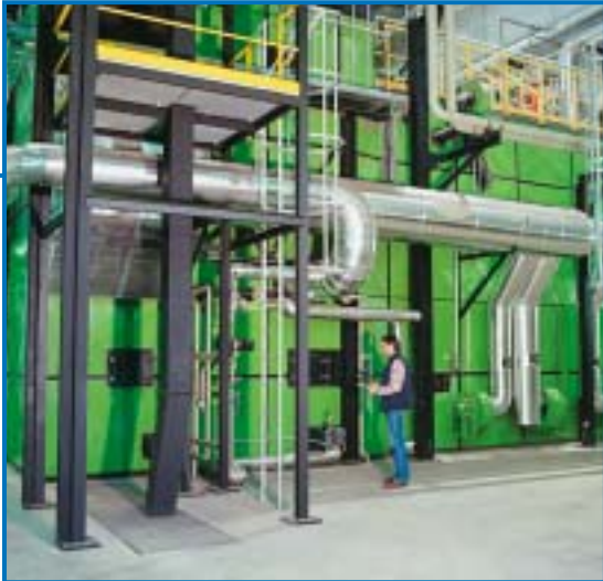
The biomass-boiler in Bystřice nad Pernštejnem, Czech Republic
