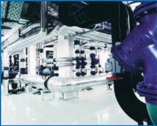
Part of the heating and cooling station
