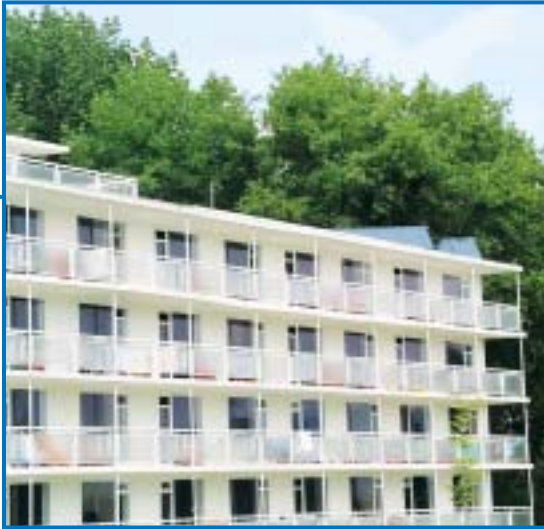
Hotel Delta in Burgas, Bulgaria, with solar collectors mounted on the roof
