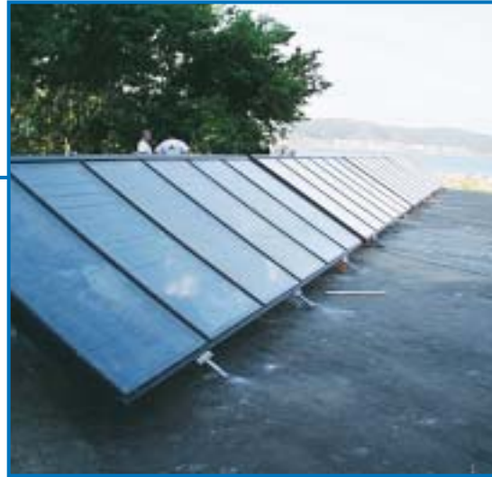
100.8 m 2 solar collector area on the flat roof of the hotel
