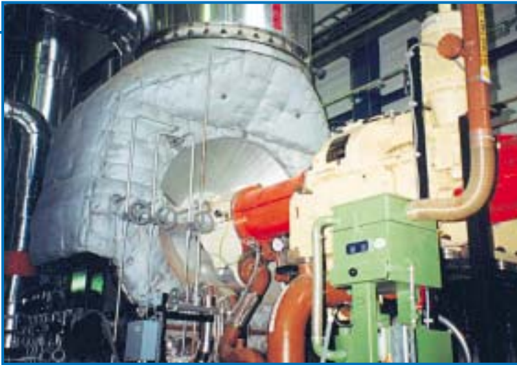
Inside view: One of the two gas turbines with a nominal output of 16 MWe
